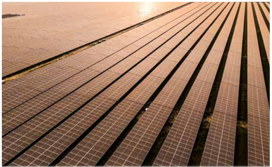
Figure 1: Utility scale solar installation by Pashupati Renewables, symbolizing Nepal's emerging solar era.
