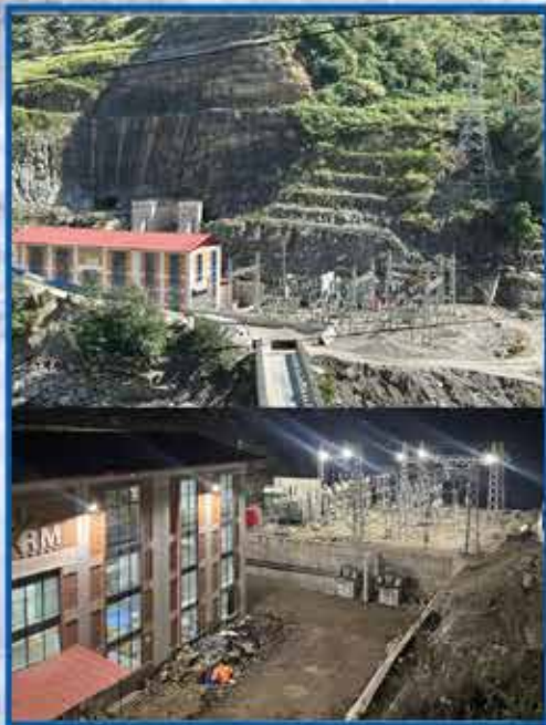
Langtang Khola Hydroelectric Project (20 MW+ 10 MW)
